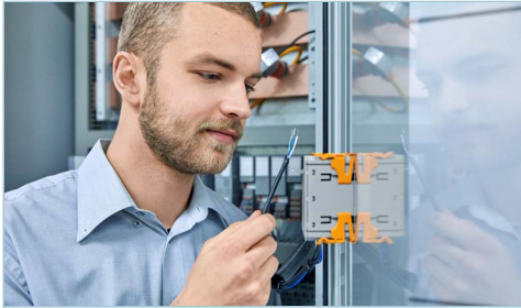
Fast wiring and configuration
